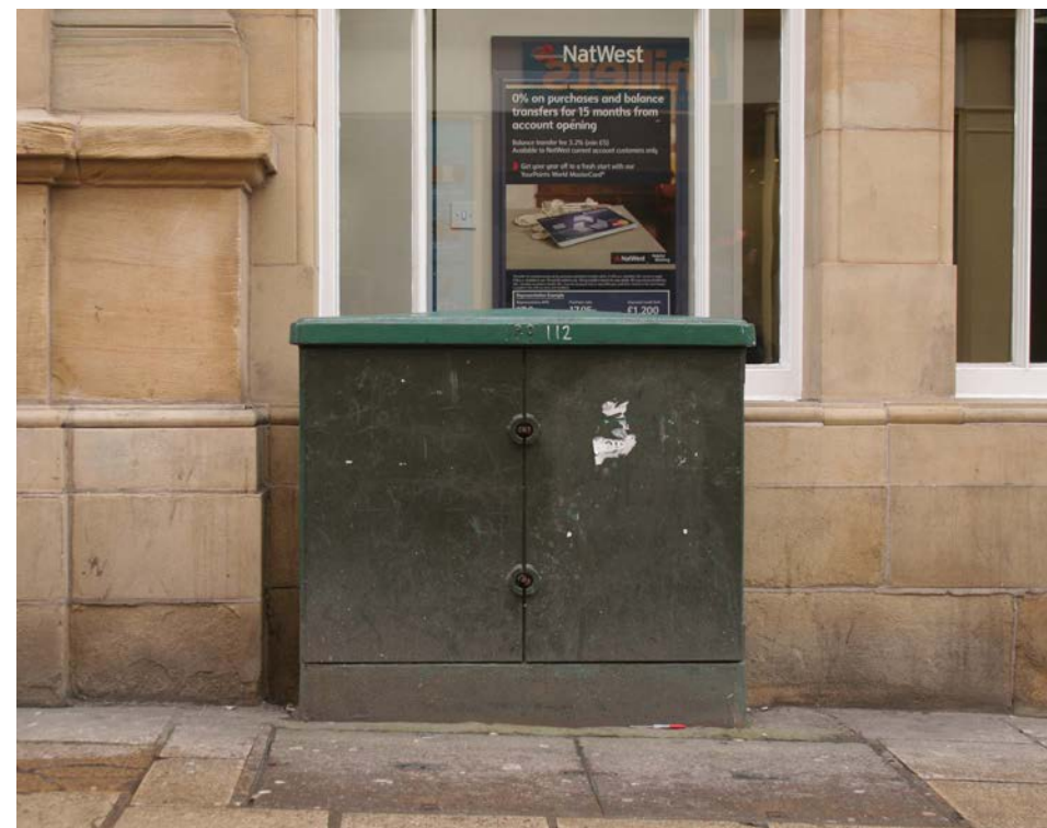
Green cabinet contrasting poorly with warm Magnesian limestone on Market Street in the centre of the footstreets. Gloss black would improve this although relocation would be preferable, where technology changes.
