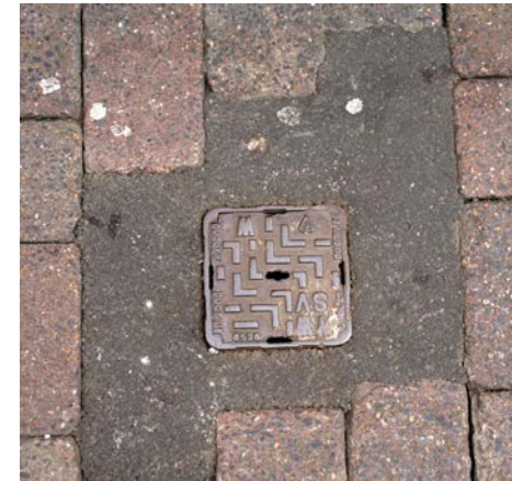
An extremely poor example of repair work by utility contractors using cement rather than the original brick paviments
