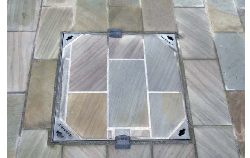
An excellently designed and laid utility inspection cover in Doncaster's cultural quarter. Note the neat jointing.
