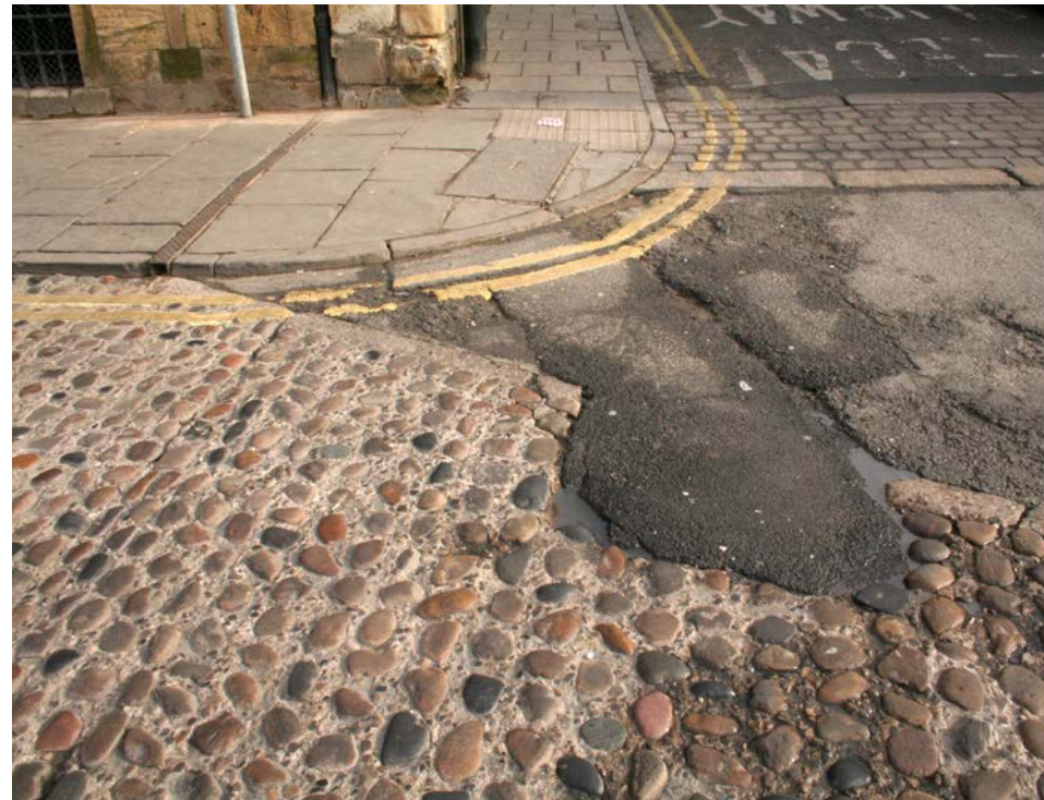
An awful utility company reinstatement of a historic cobbled surface at King's Staith
