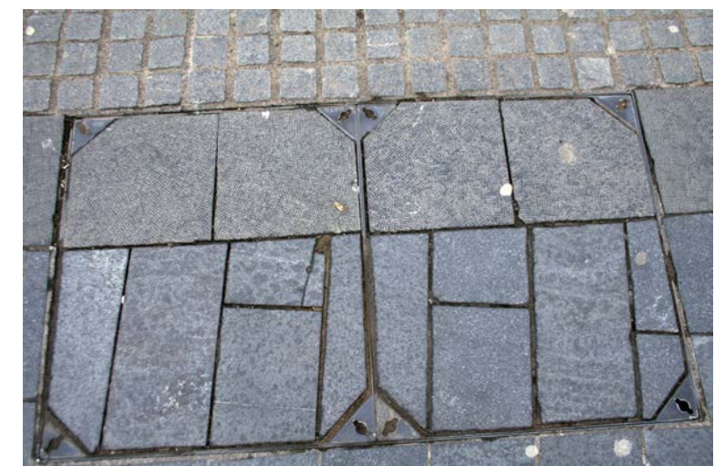
A poor example from Sheffield where more than one material has been used to infill the inspection cover
