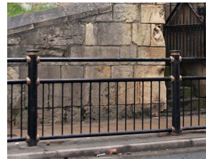
Overly ornate railings at Walmgate Bar
