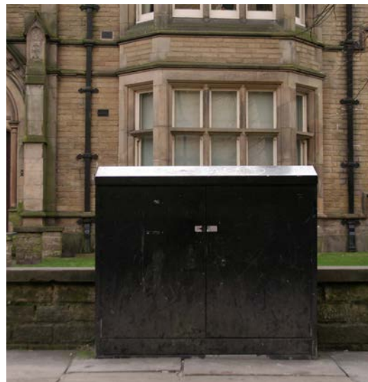
Street cabinet in gloss black, positioned against the pavement back edge on Duncombe Place. Well-positioned but in a challenging location
