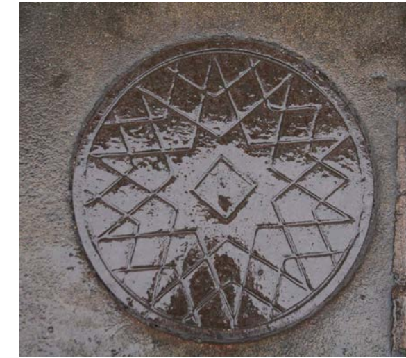
Decorative inspection cover
