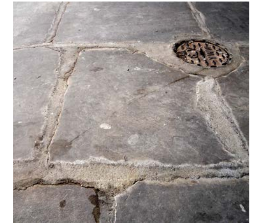
Wide joints in riven English Pennine sandstone poorly pointed with cement mortar
