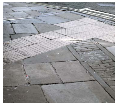
Poor use of tactile paving in King's Square where it is not really needed
