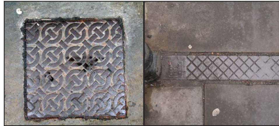
Two types of cast iron feature - on the left, an inspection cover by Dove and Sons, and on the right a cross footway rainwater channel by William Kirk.
