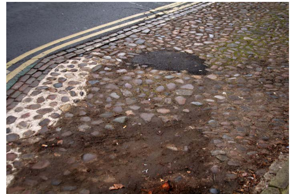
Cobbles on Blossom Street with contrasting reinstatement (white cement) and repair (asphalt) resulting in a significant visual detractor on this historic gateway street. The spacing of reinstated cobbles is also poor.
